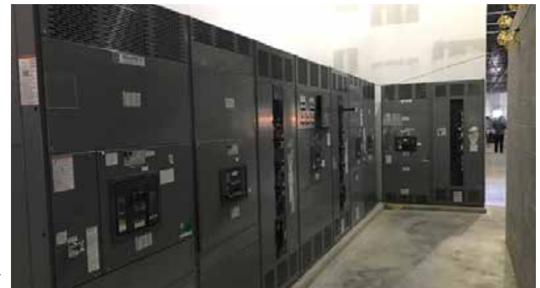
✓ 400AMP ELECTRICAL SERVICE
