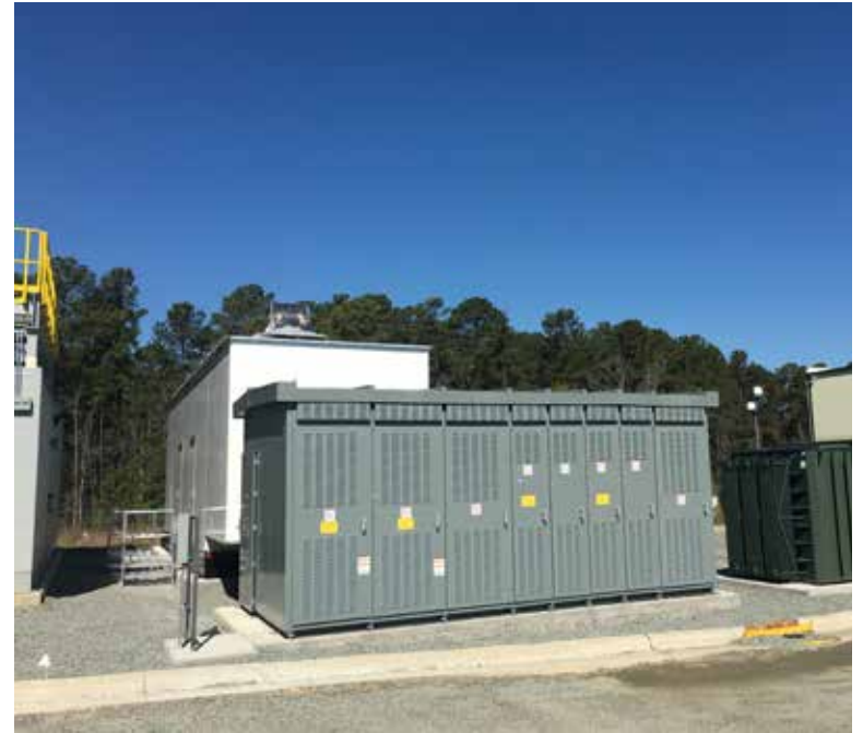
▼ DUKE ENERGY GENERATOR AND SWITCHGEAR
